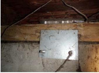
Un-finished simpson bracing in the crawlspace
