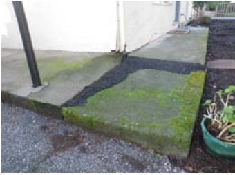
Settlement patched front walkway
