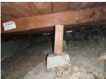
Significantly tilted post supports
