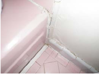
Bathtub separation and wall water damage
