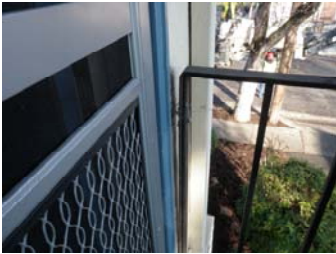
Wrought iron staircase settlement separation
