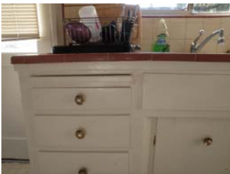
Sloping floor attribute to crowned kitchen counter / cabinet
