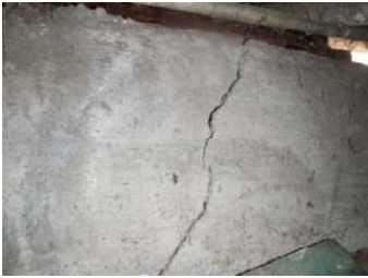
Displaced foundation cracks
