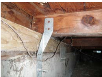
Un-finished retrofit simpson bracing in the crawlspace
