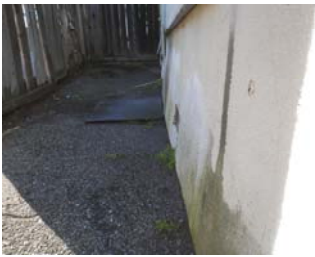
right side yard depression with drain collector
