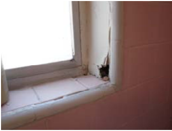
Bathroom window sill damage and expanded sill tiles
