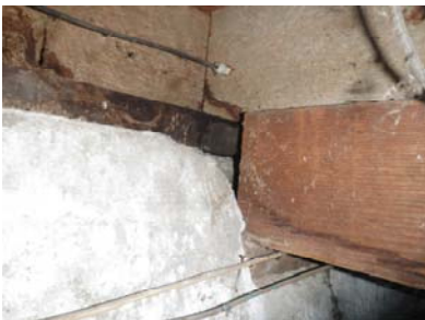
Sub structure support girder barely supported in pocket
