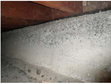
Poured concrete foundation surface spalling deterioration
