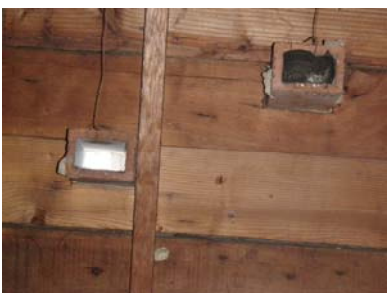
Gable vent tubes missing screen coverage
