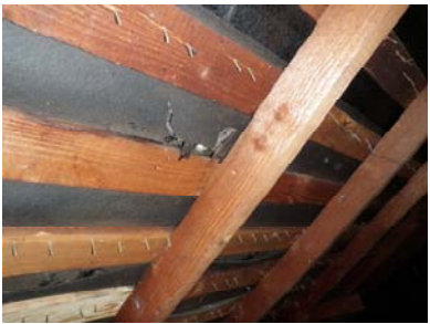
Roof felt underlayment penetration damages
