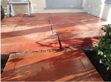
front porch settlement crack damage
