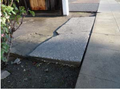
Driveway settlement and trip hazard side walk transition
