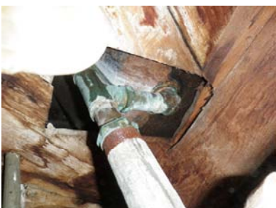
Bathtub hot / cold fixtures leaking in crawlspace during use
