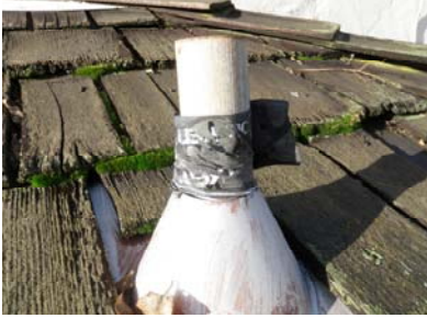
All vent jacks poorly sealed
