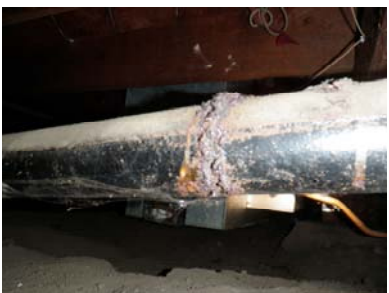
2" Cast iron drain pipe corrosion deterioration and leaking
