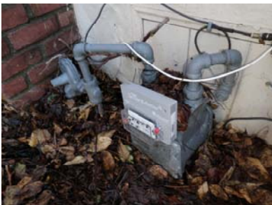
Gas meter and shutoff valve buried and not accessible
