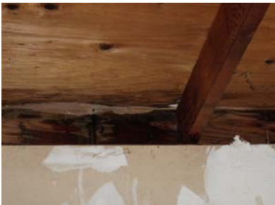
Detached garage roof structure fungus damage
