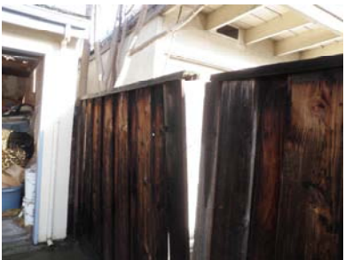
right side yard fence damage
