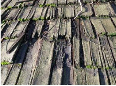
Deteriorated condition of roof wood shake coverage
